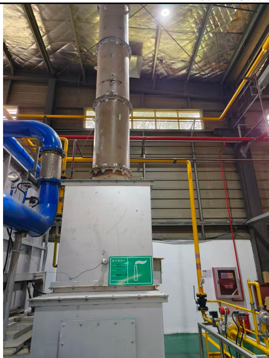
废气排放口标识牌-高温煅烧DA001
