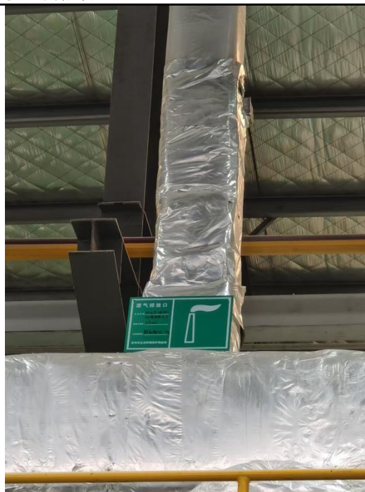
废气排放口标识牌-烘干DA006
